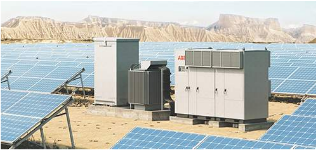
Figure 6. Power conversion station.
